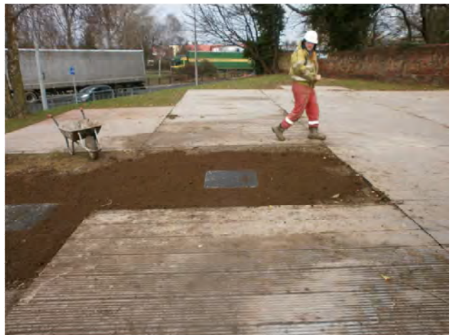
Photo 8: LDBH01 Chamber Cover, looking N towards Mytongate Junction
