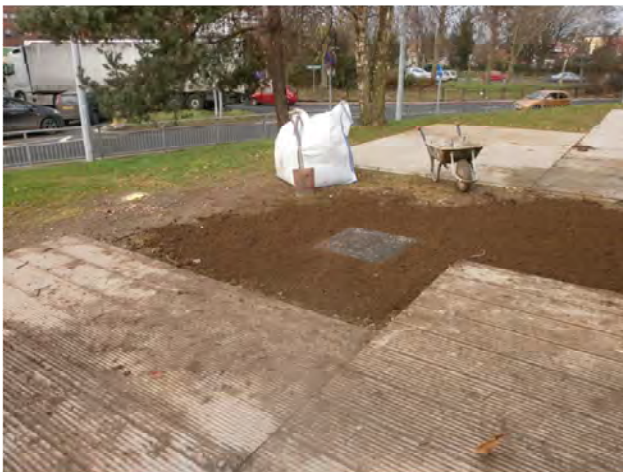
Photo 7: LDBH02 Chamber Cover, looking NW towards Mytongate Junction
