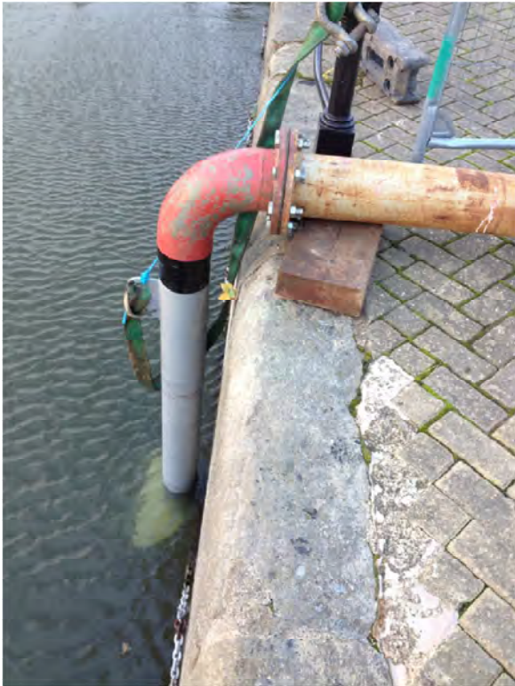
Photo 1: LDBH01 pumping test discharge point at Railway Dock, 5 Dec 13 (prior to pumping test)
